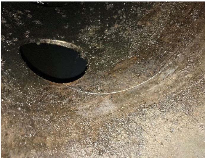
Figure 1: Acoustic pulsations can damage components in the pulsation attenuator
