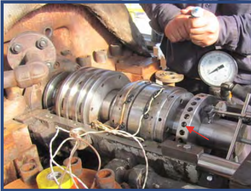
Figure 1 - The red arrow points to the turbine speed probe targets. Note the spacing of the targets relative to the target diameter.
